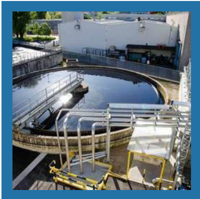
Sewage Water Treatment Plant
