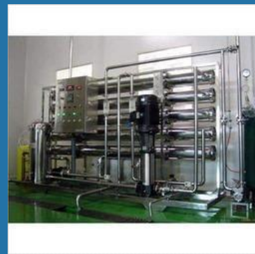
RO Plant Maintenance Service
